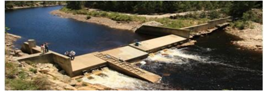
Figure 1. Keurbooms river gauging weir in August 2013 after the 2011 and 2012 flood events, showing damage to the left flank.
