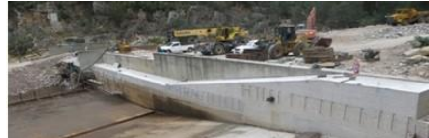
Figure 2. Reconstruction of left flank damaged wall
